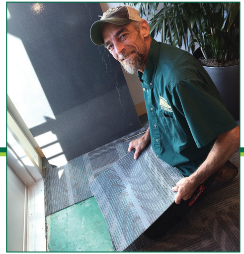
On the Job: Mark "Dana" Fussell repairing water damaged carpet following Hurricane Hermine.
