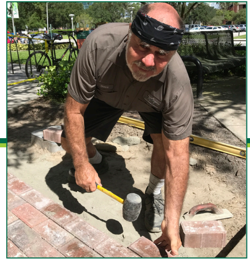
On the Job: Steve Leeds , mason, lays brick pavers at the Honors Garden in front of the Library.
