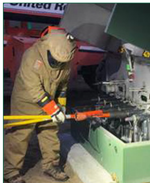
High-Voltage electrician in an arc-flash suit uses an electric meter to check voltage and make sure the phases are aligned.
