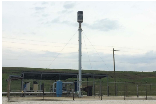
Figure 2: Landfill gas flare station
