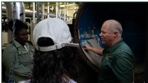
Chris Fleischer explaining the water treatment process and the effects on the chiller condenser tubes.
