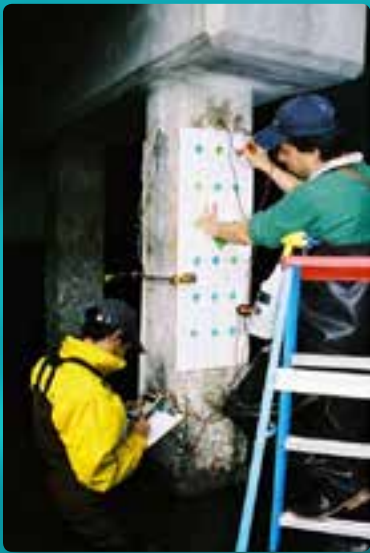
Mapping corrosion state of piles before FRP wrap
