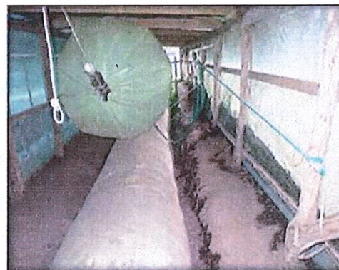
Figure 4. Anaerobic Digester and Gas Collection
